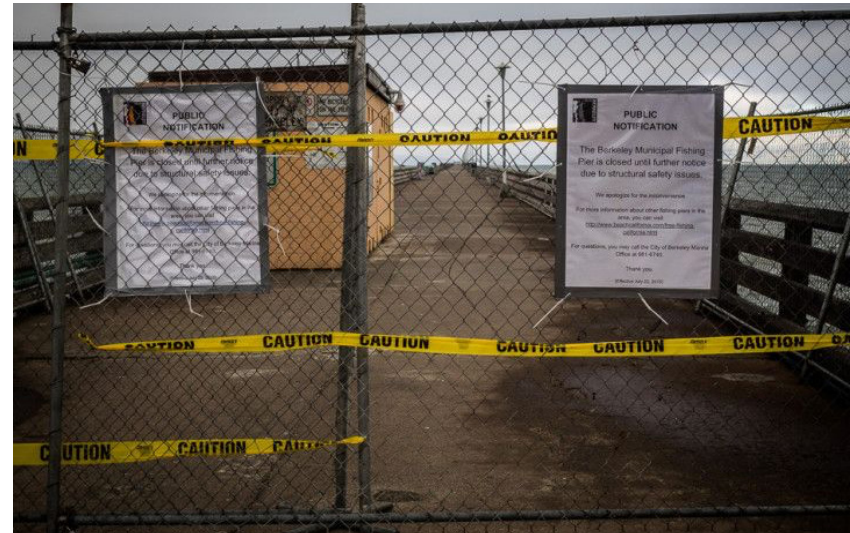
The pier is an example of deteriorated and unsafe infrastructure. Photo: Dorothy Brown
