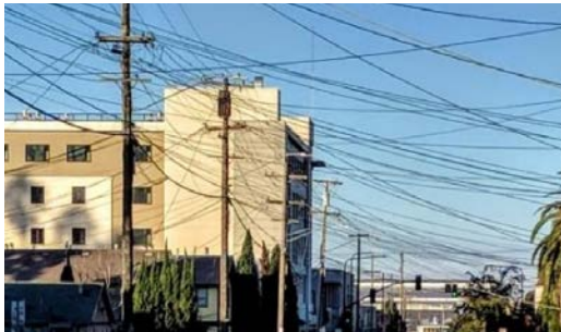
Dangerous overhead wires
