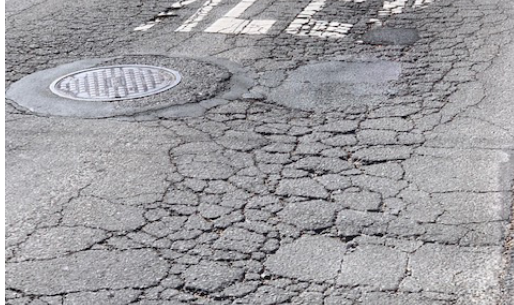
Impervious, deteriorating surface
